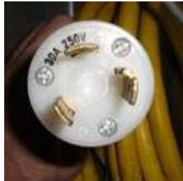
220 volt, 30 amp single-phase Connection
