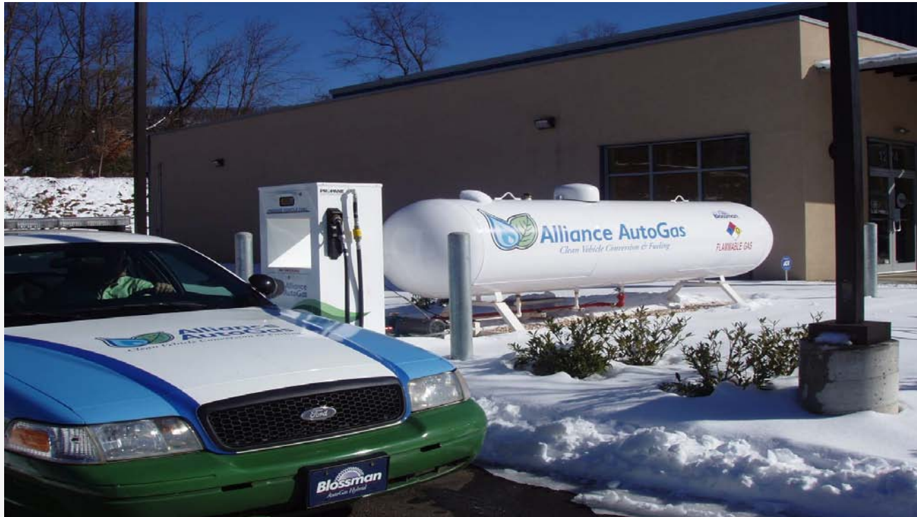
Alliance AutoGas Public Fueling Station at German Motor Werks in Asheville, NC
